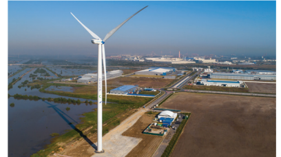
Wind Power Deep C II Hai Phong
